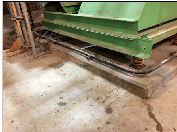
Cracks in Existing Fan Equipment Pads
