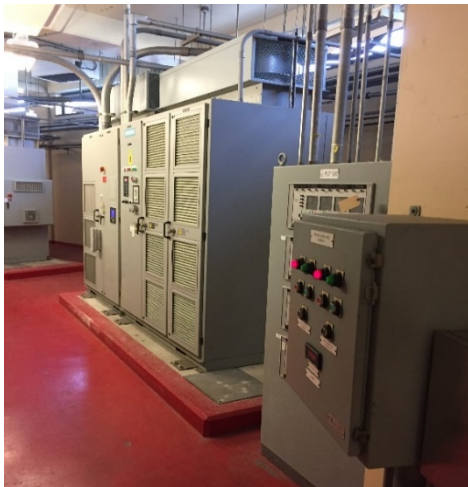
SSPS Pump Variable Frequency Drive
