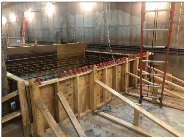
Odor Control Fan 4 Equipment Pad
