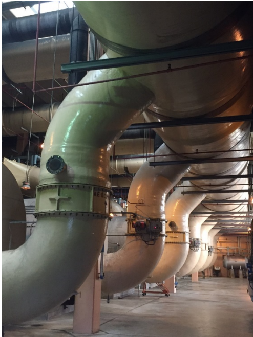
East Odor Control Carbon Room
